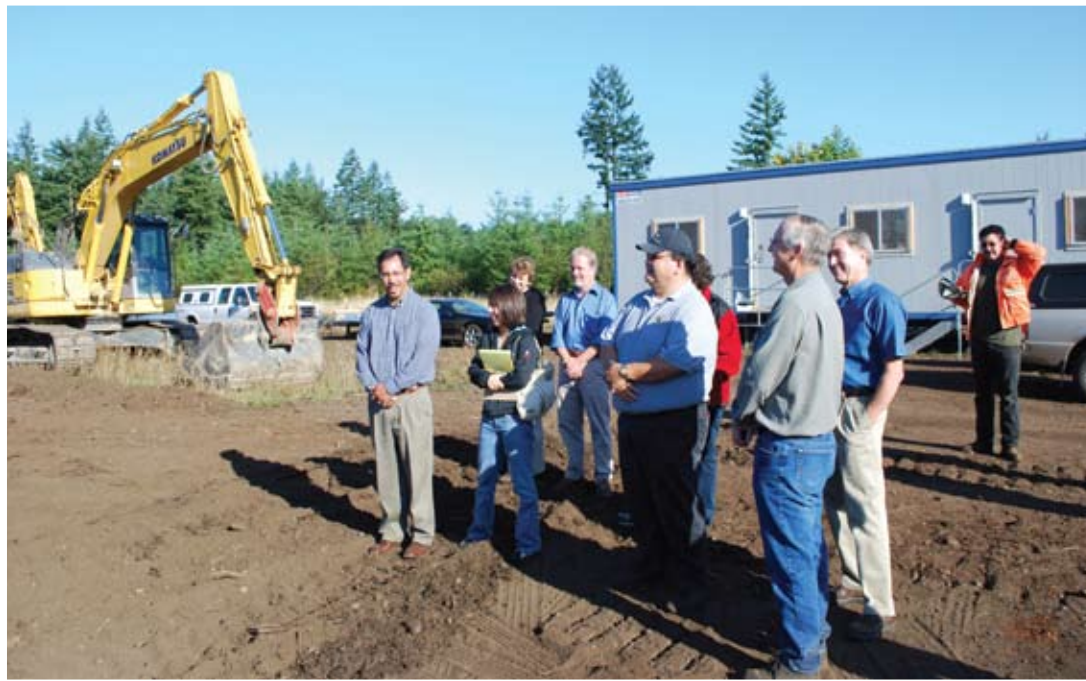
Tribal Chairman David Burnett (left), Vice Chairman Don Secena (with cap), tribal staff and construction crew wait for a blessing of the land by Dan Gleason, Sr., for the tribe's new community center.
