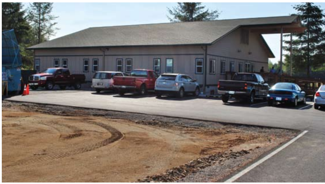
The beautiful, new Chehalis Tribal Enterprises building was constructed from five pre-built trailers. It stayed on budget and saved the tribe money. Construction of a new storage and cigarette packing plant is in the process.
