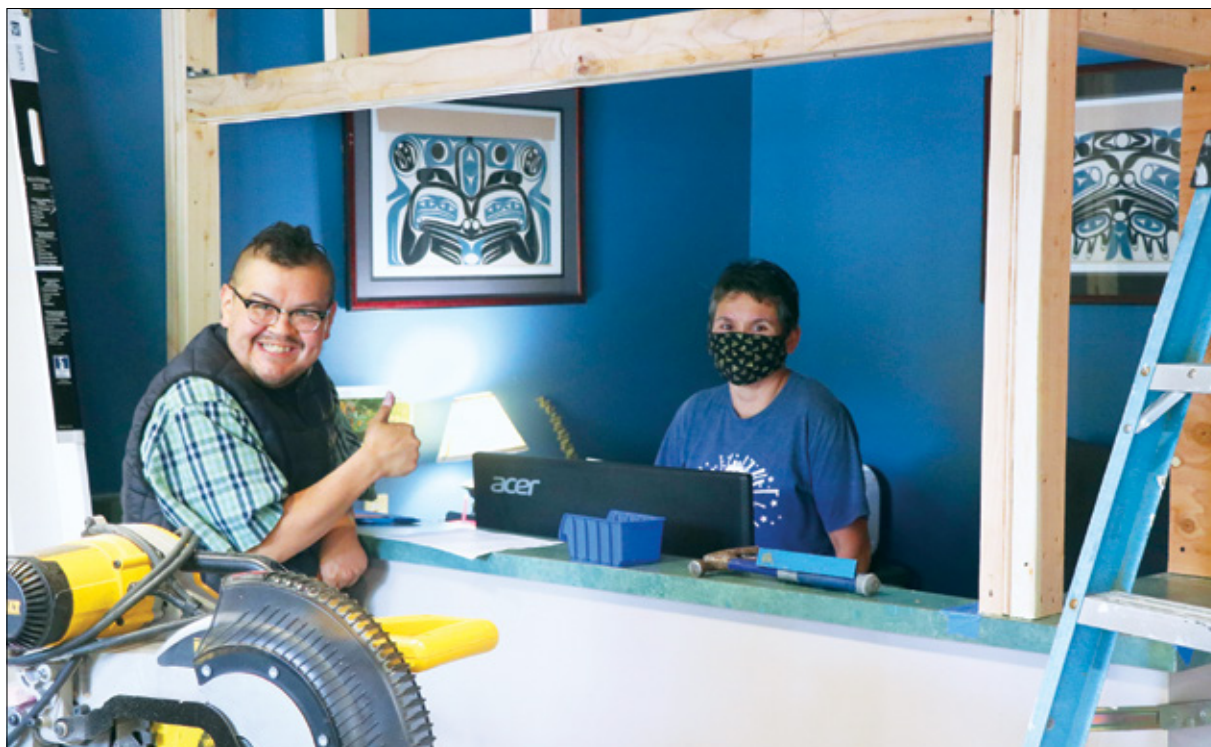
Chehalis tribal building were modified by Facilities and Maintenance crews to help prevent virus outbreaks.
